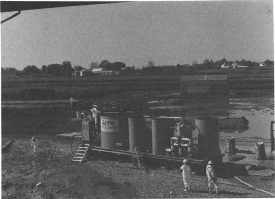
Fig. 2. Photograph of independent physical/chemical treatment unit used for contaminated runoff treatment at Seymour, Indiana.
